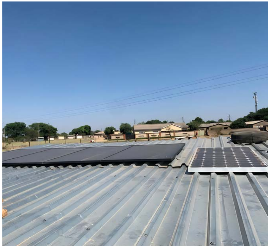
Solar panels used to pump water from boreholes as a clean, renewable and affordable option, Kadoma, Zimbabwe, S Nyoka, 2023.
