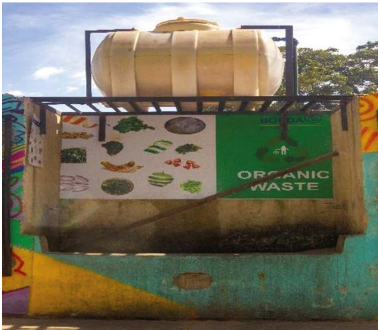
Methane producing biodigester used by Lusaka Boys Secondary School for cooking, lighting and fertilizer, Lusaka, Zambia. P Phiri, 2023.
